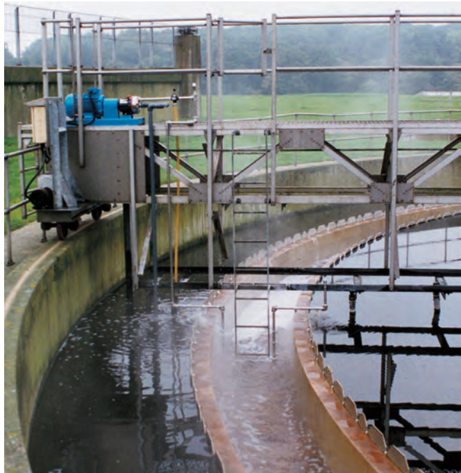
Hydra-Cell operating in a wastewater treatment facility.
