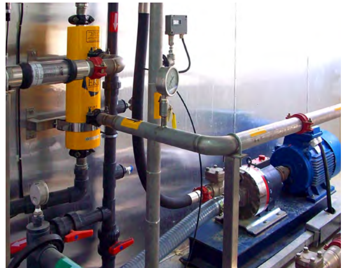
RO recovery device.
