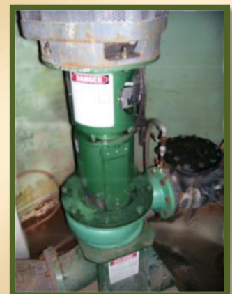
1 of 2 retrofit Vaughan pedestal Chopper pump with older motor
