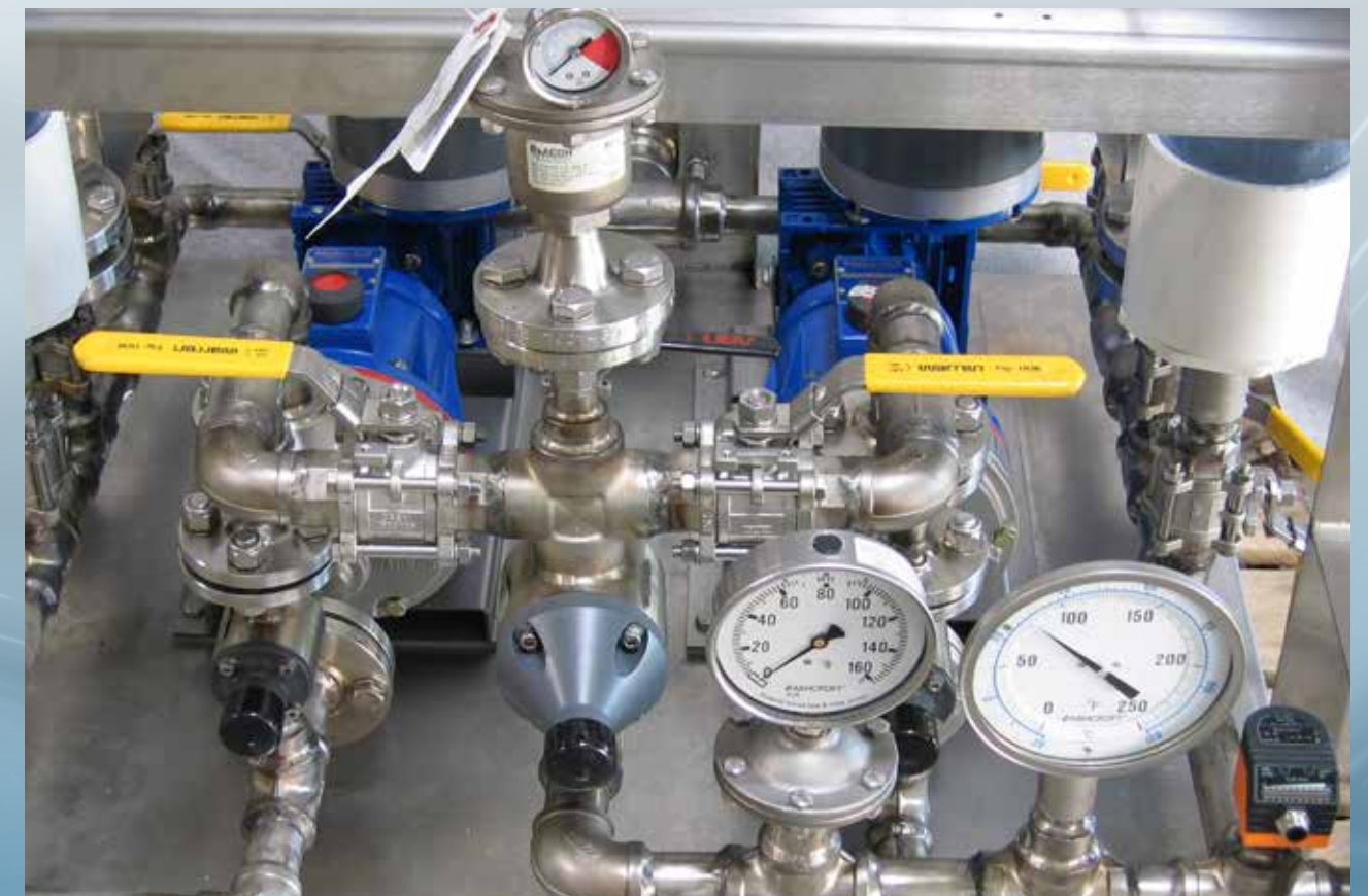
Polymer dosing for water treatment
